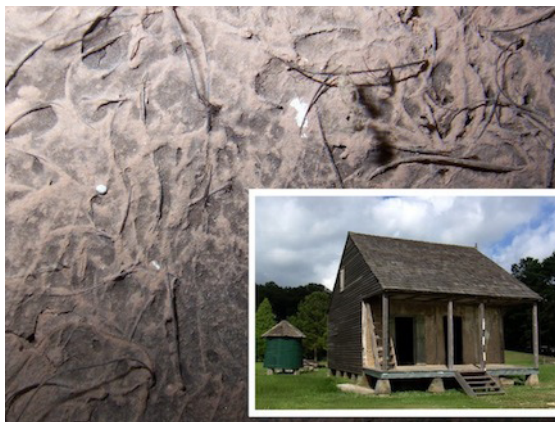
Bergeron House, Rural Life Museum, Baton Rouge, LA showing bousillage exposed on front elevation, with detail of interior surface of bousillage, Yucca House, Melrose Plantation, Melrose, LA in background. Photos by Laura Blokker, 2008.
