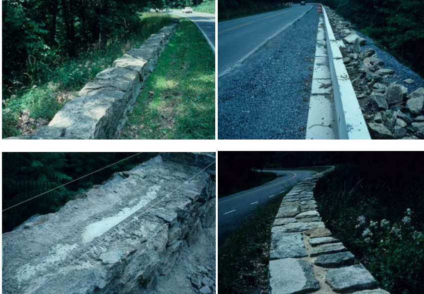
(left to right) Historic stone barrier walls (upper left) along the National Park Service Skyline Drive in Shenandoah National Park, Virginia, constructed during the 1930's, did not meet modern crash standards. The stone walls were dismantled, a concrete core (meeting modern crash requirements) was inserted; the original stone was used to face the core. The completed wall (lower right) closely resembles the historic wall while providing an enhanced safety feature. Paul Daniel Marriott
