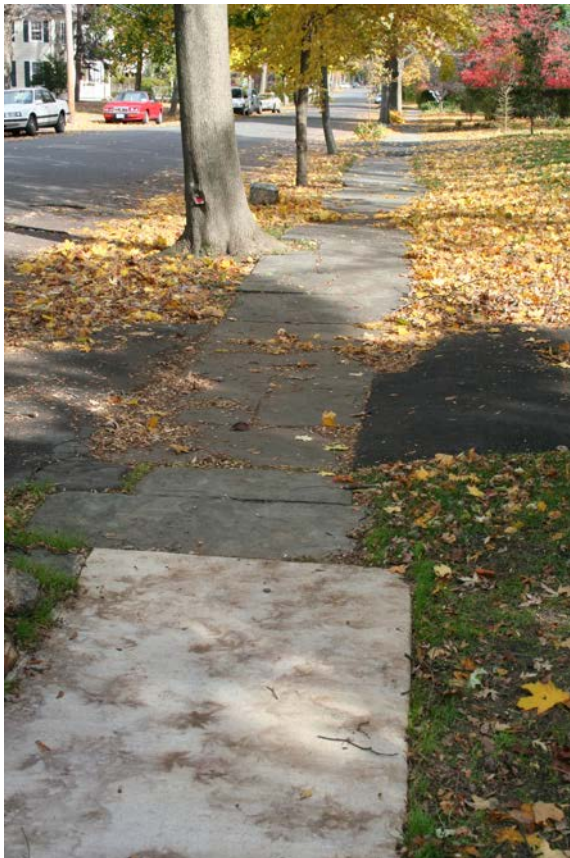
Historic stone sidewalk pavements in Rhinebeck, New York have been poorly patched with concrete (foreground). The color, texture and feel of the concrete is inappropriate to the historic district. Paul Daniel Marriott
