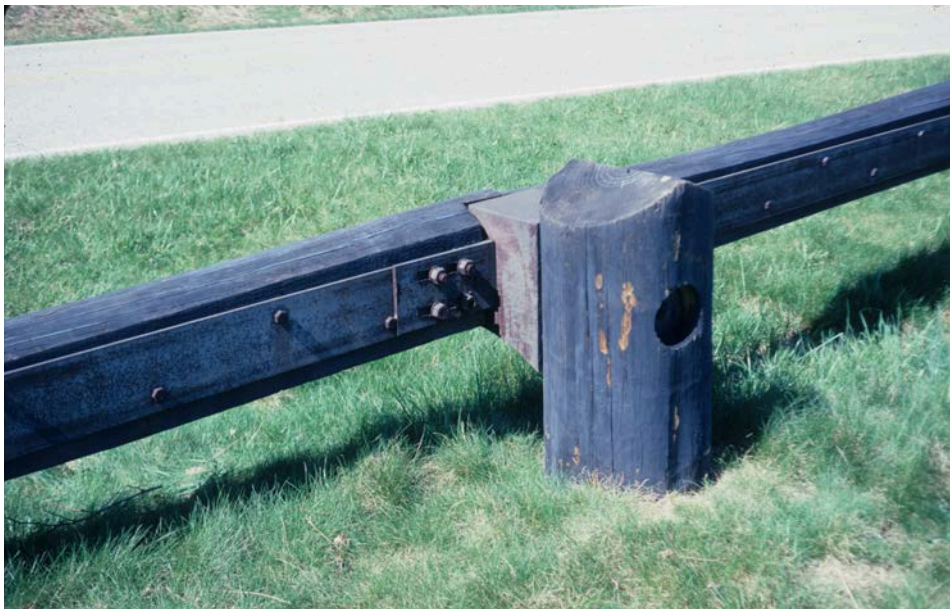
New guardrail on the historic Skyline Drive in Shenandoah National Park reflects the historic design of the original wood posts and rustic rails of the 1930s with the addition of steel-backing for reinforcement and “block-outs” at the posts to prevent “snagging” (preventing the wheels of an errant vehicle from striking the post). The barrier has been crash tested and meets federal guidelines for guardrail design. Paul Daniel Marriott
