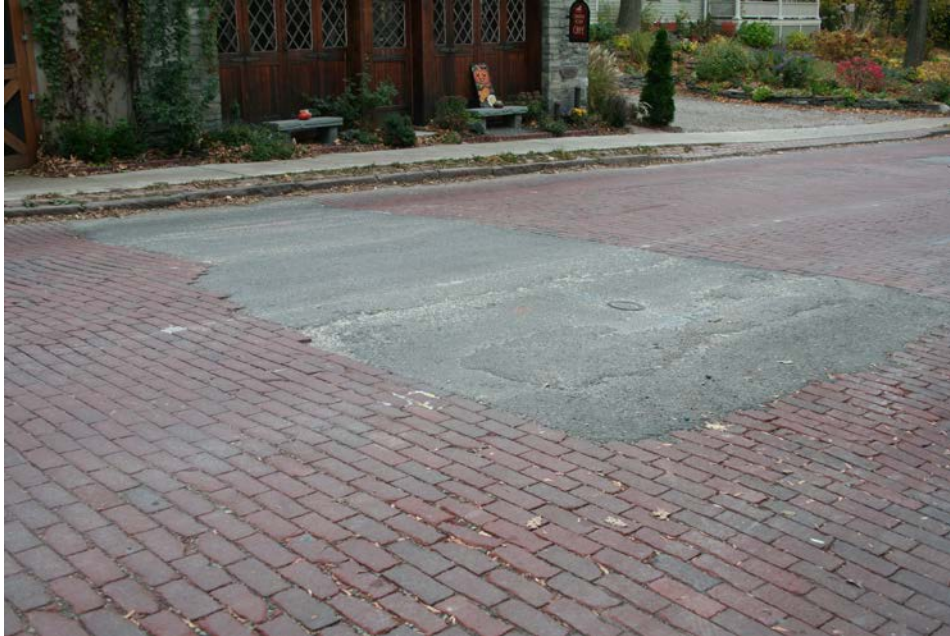
Repair of this historic brick street would be an example of preservation. Paul Daniel Marriott
